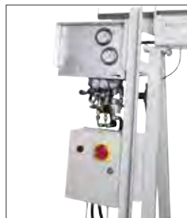
Detail of the control panel.
